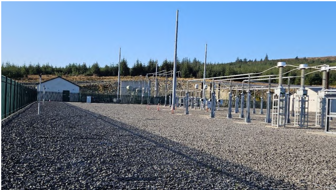
Plate 4-3 110kV Electrical Substation
